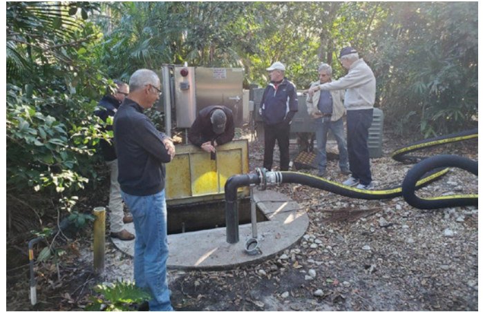
WILTON CRESCENT: Test of new Bypass Pumper
