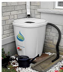
Installed Rain Barrel
